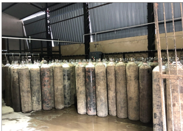
The Oxygen Manifold in Trauma Building
