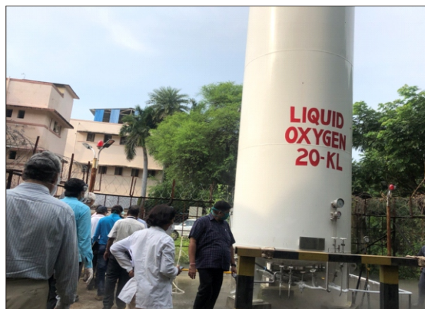
The 20 KL Oxygen tank in Main Building
